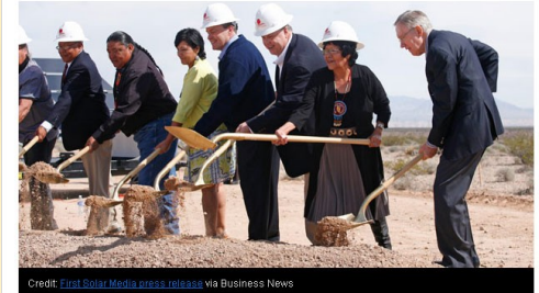
Signaling the first day of construction of the Moapa Southern Paiute Solar Project, which is about 20 miles from the Bundy homestead in Bunkerville, Nevada, Sen. Reid joined representatives from the Moapa Band of Paiutes, executives from First Solar, Inc. and the Los Angeles Department of Water for the groundbreaking ceremony on March 21.
